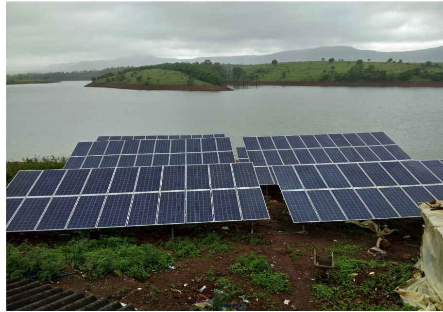
50HP Solar Water Pump at Takawe, Pune
