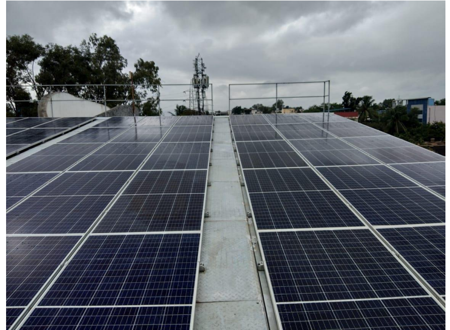
50Kw Solar On Grid Power Project at KPPL, Bhosari Pune
